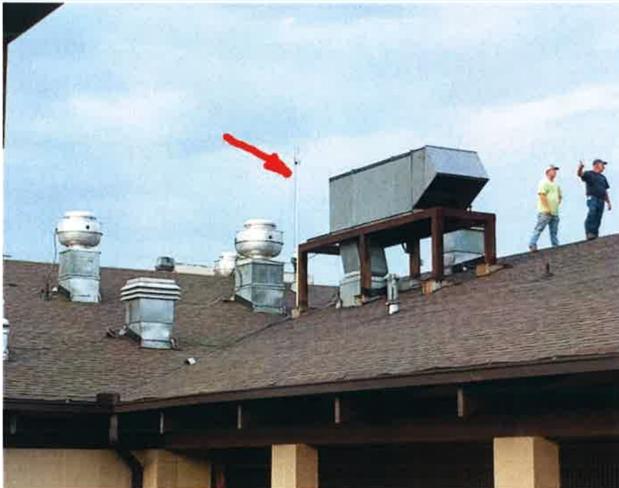
Electrical Conduit Mount attached to AC unit.
