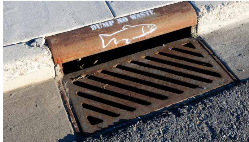
"Dump No Waste" Storm Grate
