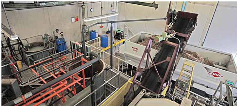
Ishpeming Area Wastewater Treatment Facility
