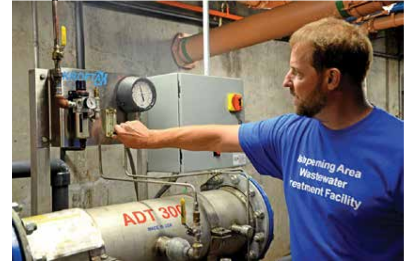
Ishpeming Area Wastewater Treatment Facility
