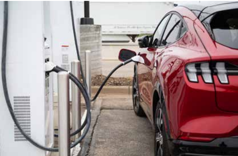
An EV Charging Station
