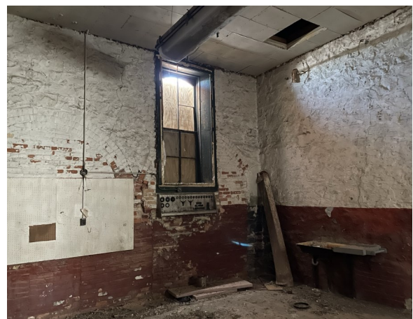
Northwest Corner Intake Room
