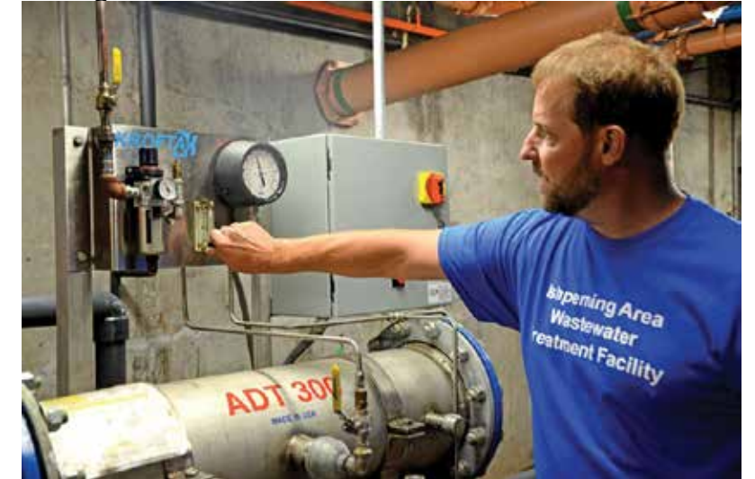
Ishpeming Area Wastewater Treatment Facility
