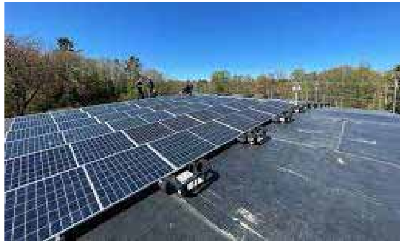
Solar Panels on roof in Negaunee Township
