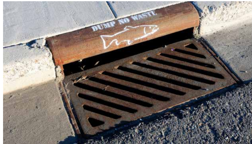
"Dump No Waste" Storm Grate
